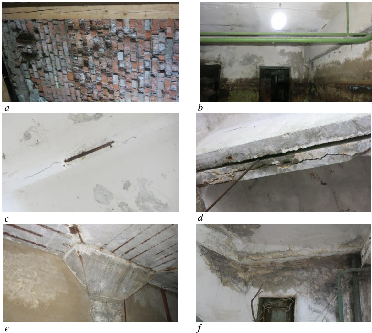
Fig. 1. 1. Degradation of structures of buildings of the former Modul plant in Uzhgorod: a – destruction of the masonry walls of the staircase made of brickwork to a depth of 50 mm in Section 2 from periodic freezing and thawing; b – traces of flooding of the shelter to a height of 2 m in the basement of Section 1 (carbonization of concrete and reduction in concrete strength); c – cracks along the edge of the floor slab on the third floor of Section 2 (corrosion of the working reinforcement in the edge of the slab); d – cracks in the rib of the floor slab on the second floor of Section 2 (destruction of the protective layer of concrete, carbonization of concrete, peeling of the protective layer, corrosion of the reinforcement of the floor slab and capital); f – periodic flooding of the shelter in the basement of Section 2, resulting in the appearance of damage shown in Fig. 1 a–f
