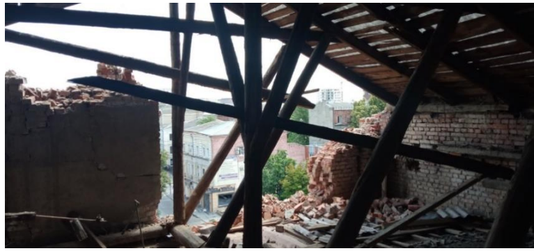
Fig. 13. Damage to wooden roof structures caused by the explosion shock wave
