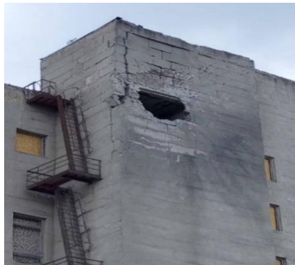
Fig. 7. Mechanical destruction of building structures in the elevator shaft by an explosive delivery device (the explosive device did not detonate)
