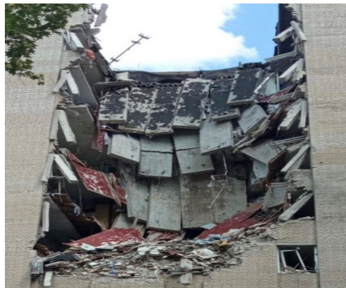
Fig. 9. Destruction of the building's structure due to an explosion inside the building
