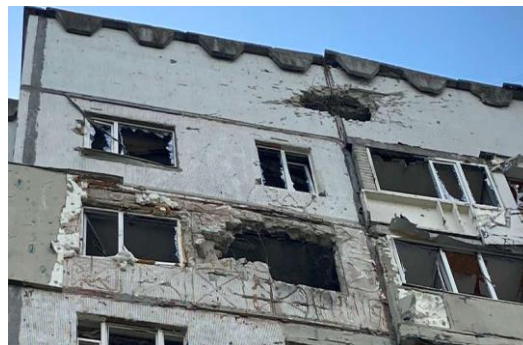
Fig. 8. Panel building structures damaged as a result of the explosion shock wave and the impact of the explosive delivery device (the explosion occurred inside the building)
