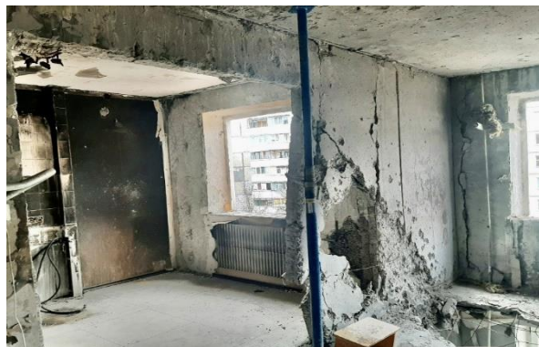
Fig.12. Destruction of floor slabs, wall panels, and panel connection joints in a residential building
