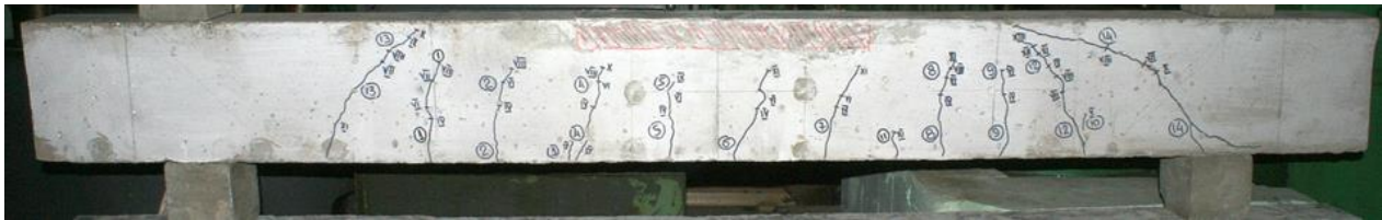
Fig. 3. Cracks in the sample RCD3
